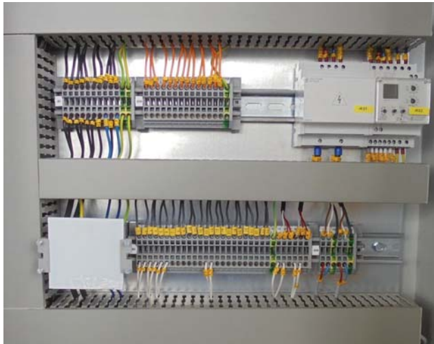
Insulation monitor of the type RN 5897 from the VARIMETER IMD series by Dold in the control cabinet of a current wind turbine.
