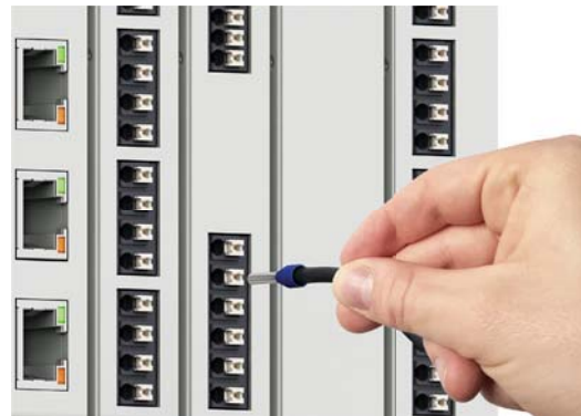
The push-in-clamps used have a test point allowing for quick diagnosis.
